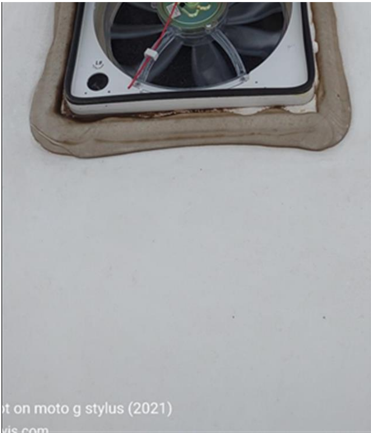
Powered Roof Vent
