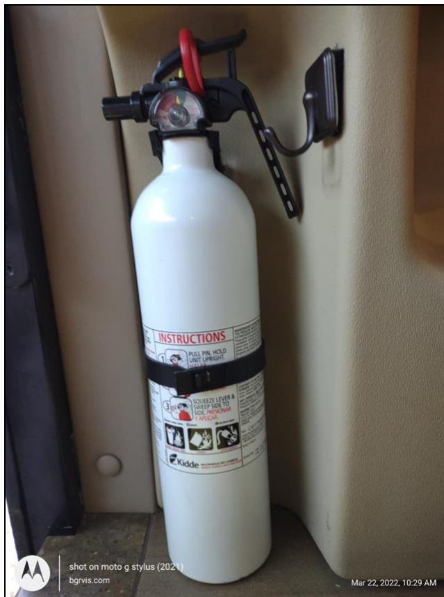
Fire Extinguisher 10 BC
