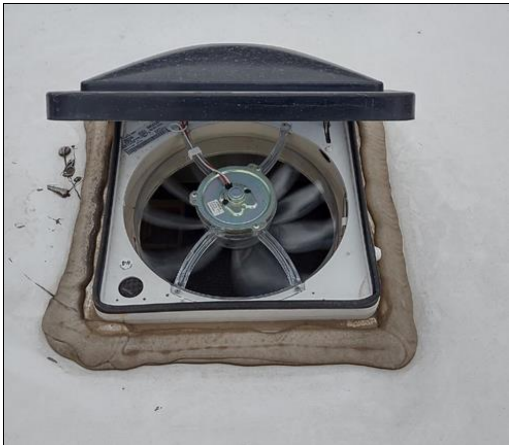
Powered Roof Vent
