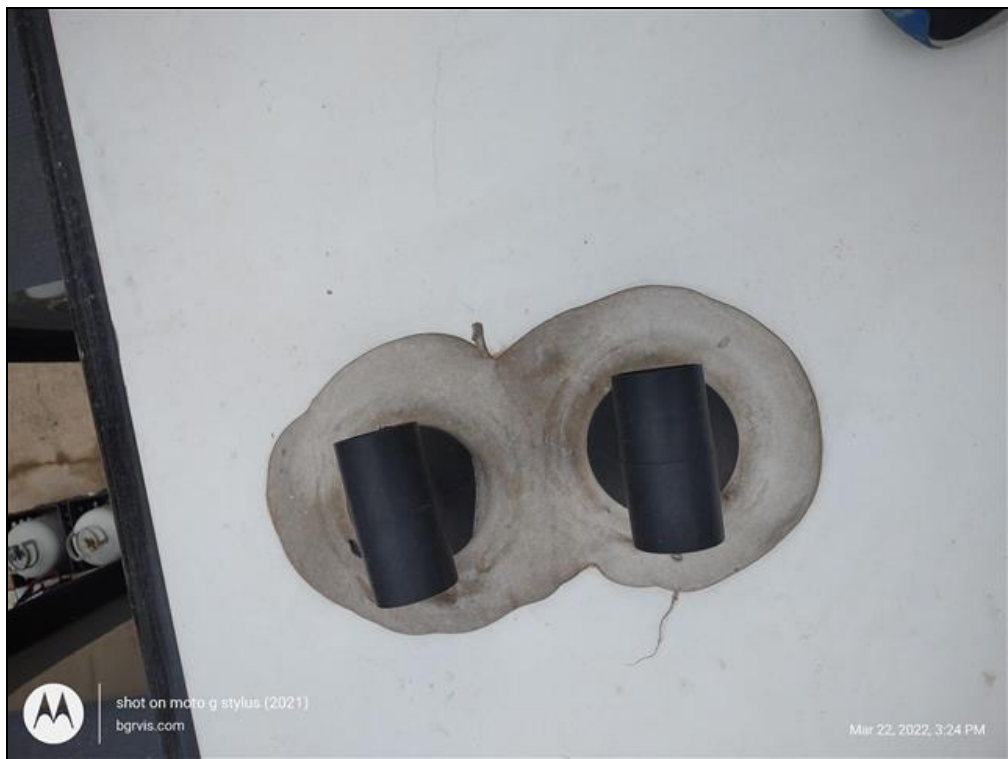
Plumbing Vent Covers
