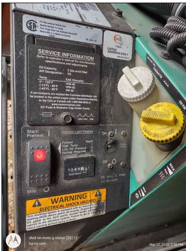
Generator control panel
